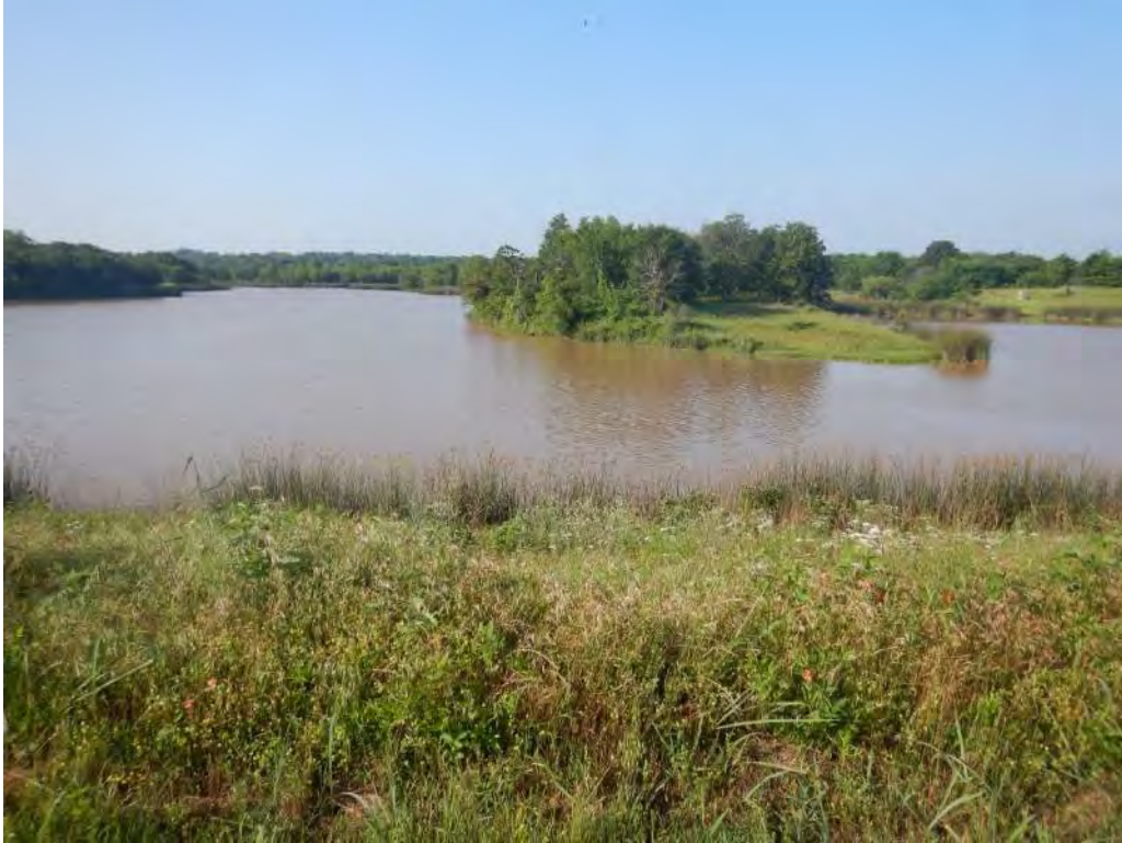
Photo 1. View looking south towards Little Wewoka 12 Reservoir from the existing dam crest.
